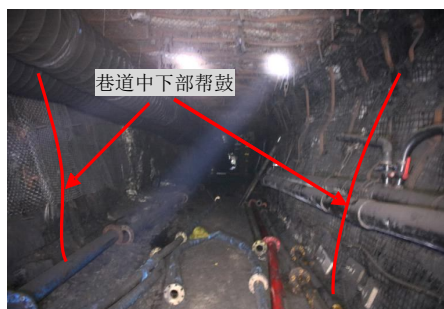
图 18 巷道围岩变形 Fig.18 Deformation of rocks surrounding roadways
